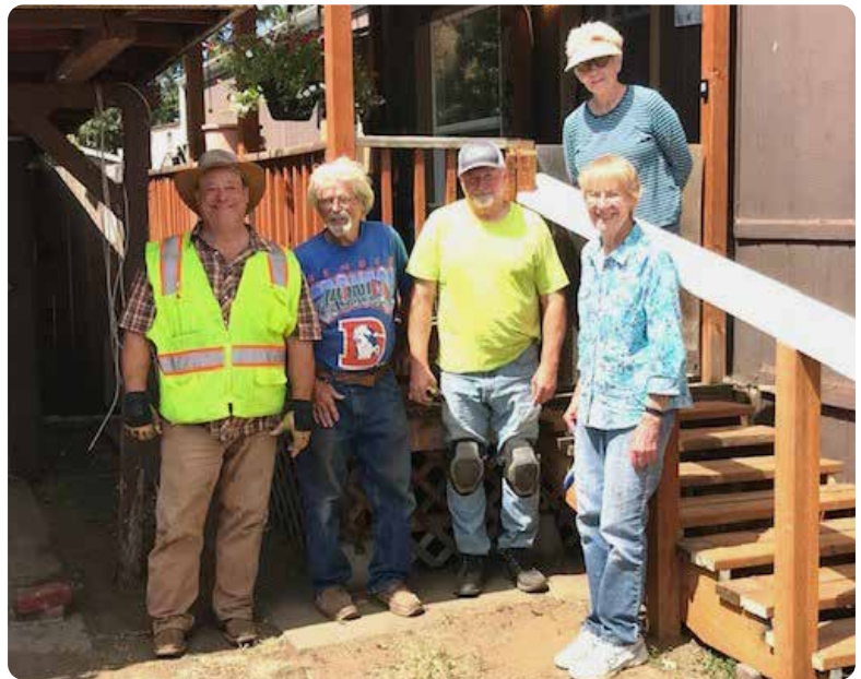
Providence and community partners build new steps for local resident after extensive surgery.
